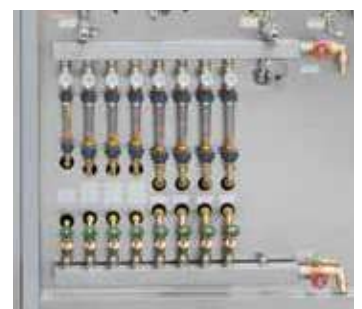
Cooling water distribution
